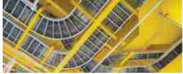
PERMANENT CONSTRUCTION CABLE TRAY
