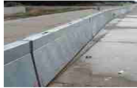
ROAD SAFETY TEMPORARY BARRIERS
